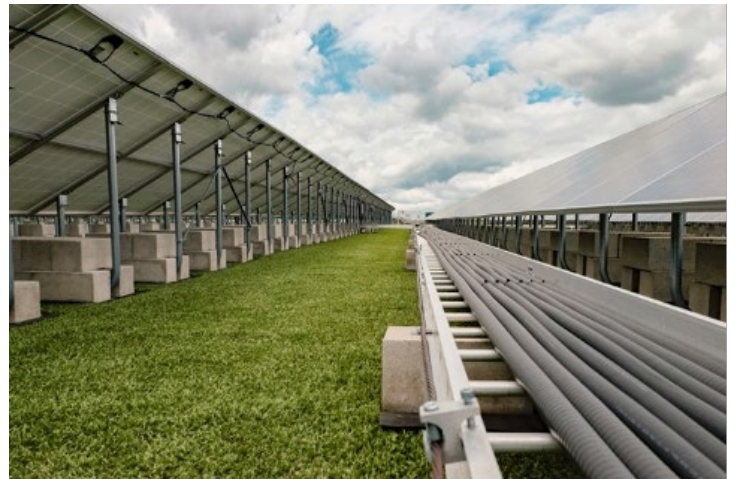
Solar panels operate free of dust, glass clippings and damage from mowing equipment.
