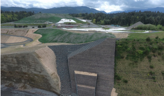
Refuse still remains in one of the slide slopes on the bluff but is stabilized by a large MSE wall embedded with survey targets to track any movement.
