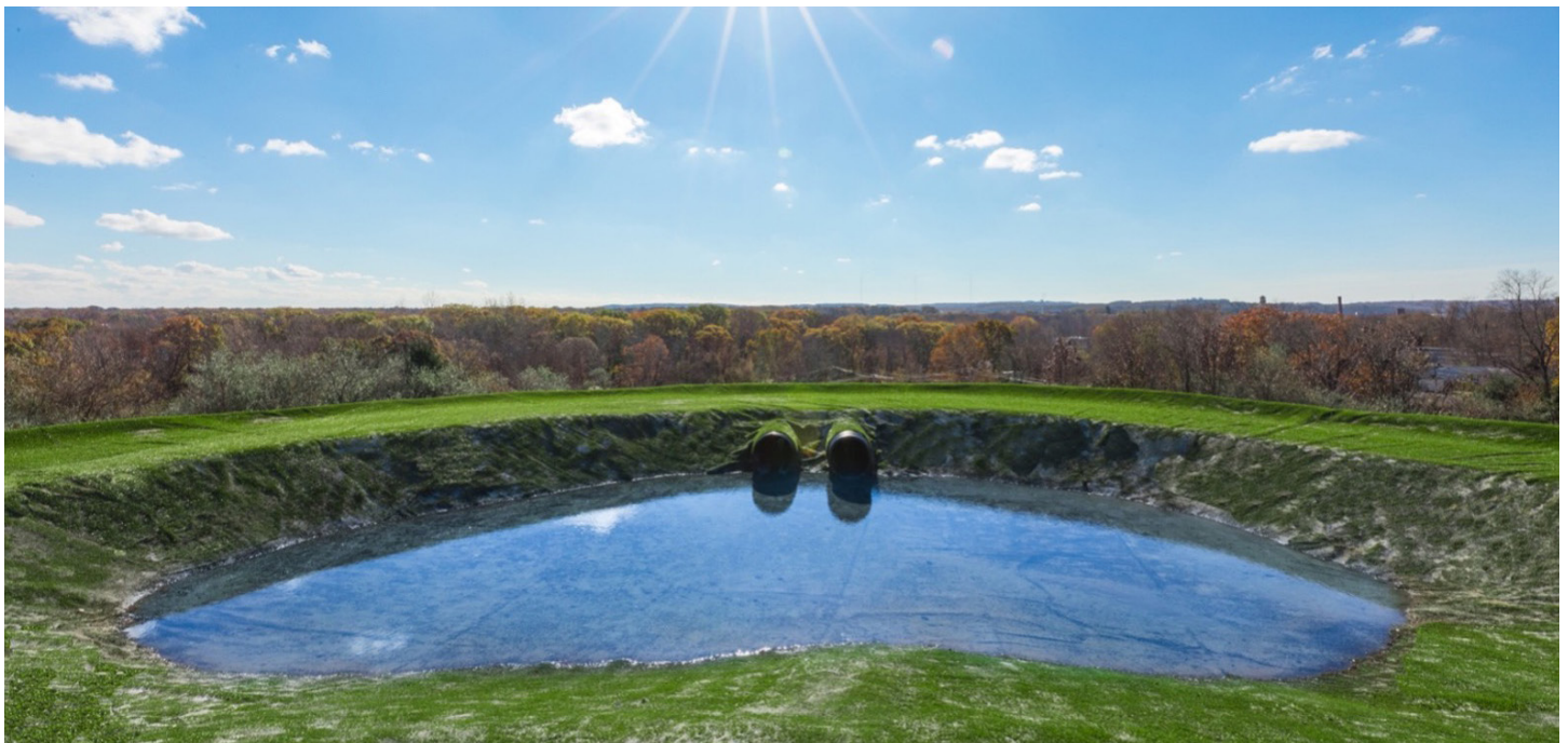
This drainage pond is lined with HydroBinder®, a cementitious infill, used in stormwater applications. The runoff contains no sediment so water leaving the site is much cleaner and safer.
