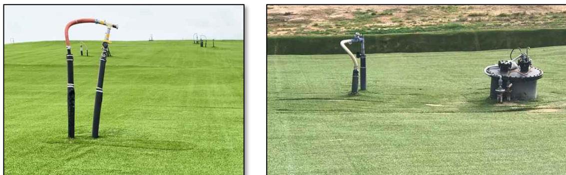
Figure 7-2. ClosureTurf Integrated with Landfill Gas Collection System
