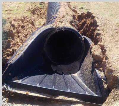
Failed Pipe Application
