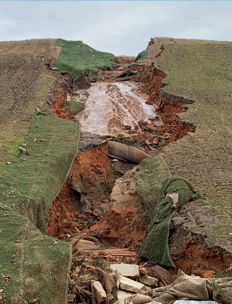
Traditional Downchute (Failed)
