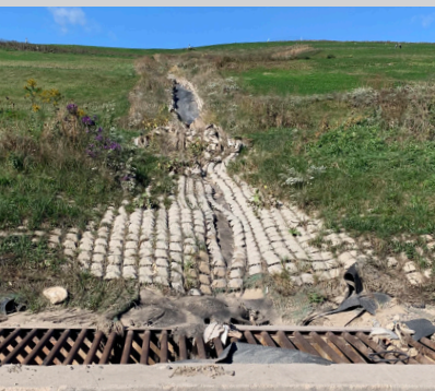
Failed Hard Armor Application
