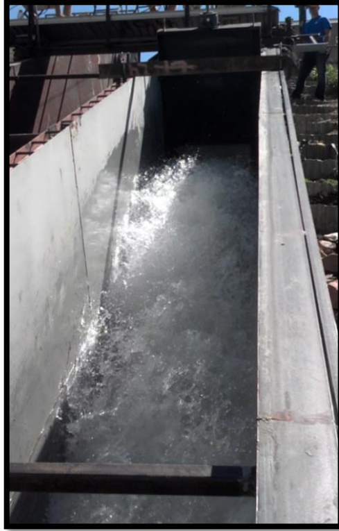
Figure 16: Pressurized “Jet” from Under the Sluice Gate Surging onto the CEST
