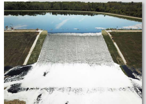
An overtopping event occurred shortly after the HydroTurf was installed. During the event, the flow rate reached a flow rate of approximately 75 million gallons per day producing an estimated velocity of 10 ft/s on the HydroTurf. It successfully resisted this velocity. A post event inspection noted no instability, damage or erosion.
