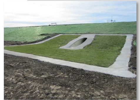
HydroTurf was used in lieu of articulated concrete blocks in the outfall and inlet structures.
