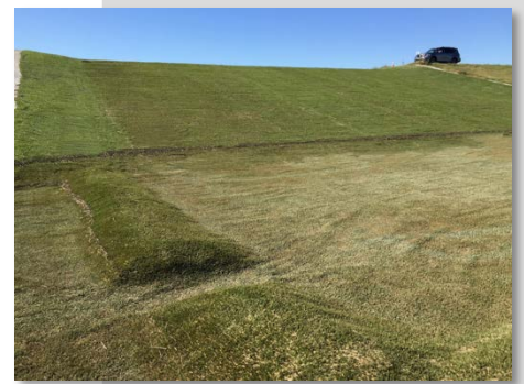
Up-close view of the HydroTurf in the dam spillway and stilling basin.
